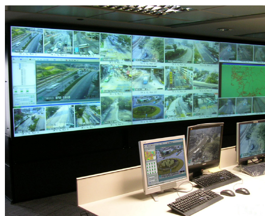
Hong Kong's Traffic Monitoring Centre
